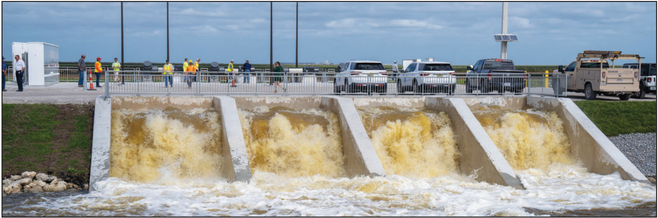
Turning on the Pumps at the EAA Reservoir Project's Stormwater Treatment Area. Photo by SFWMD.
